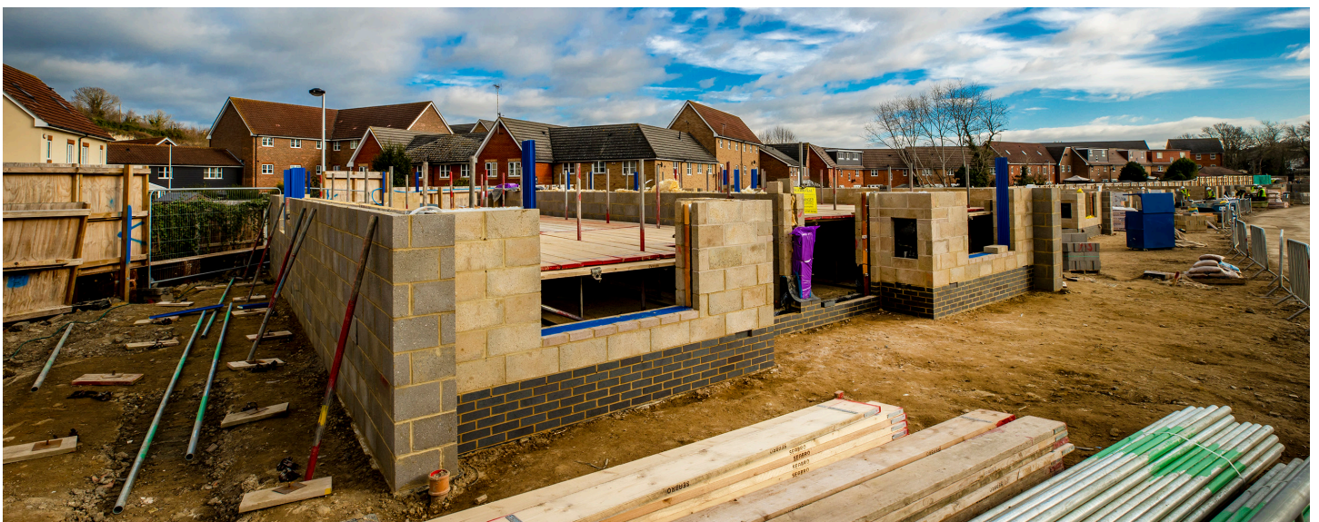
The 61 new two, three and four bedroom homes are starting to take shape.
