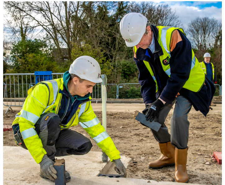
Sir Tim Laurence, Chair of PCRL, laying a brick on the first phase of homes.
